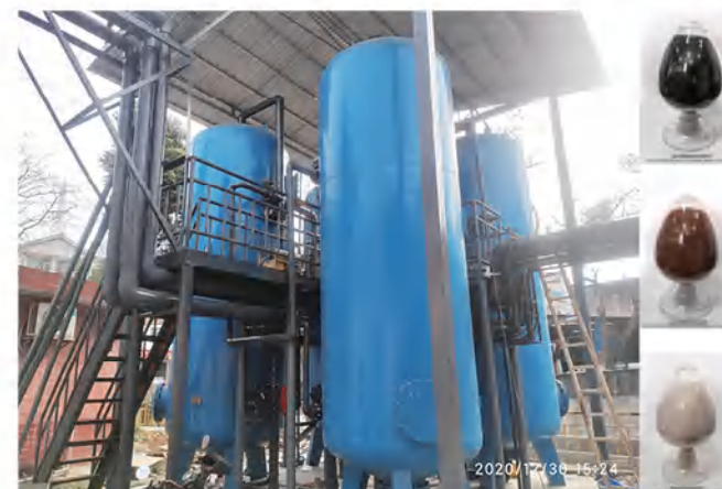
重金属废水纳米吸附深度处理工程 Advanced nano-absorption treatment project for heavy metal wastewater
