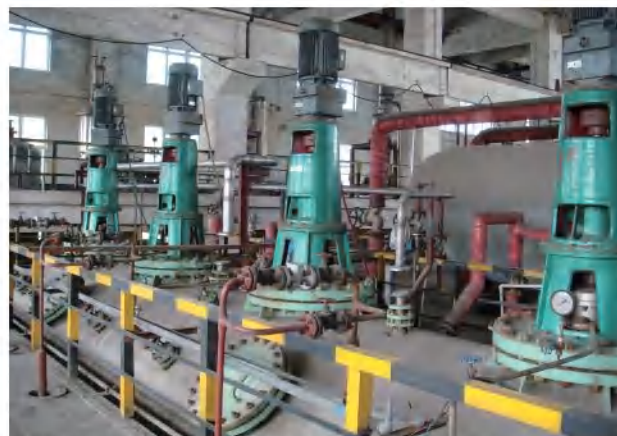
铜镍矿加压浸出精炼工程 Cu-Ni refining project with pressure leaching process
