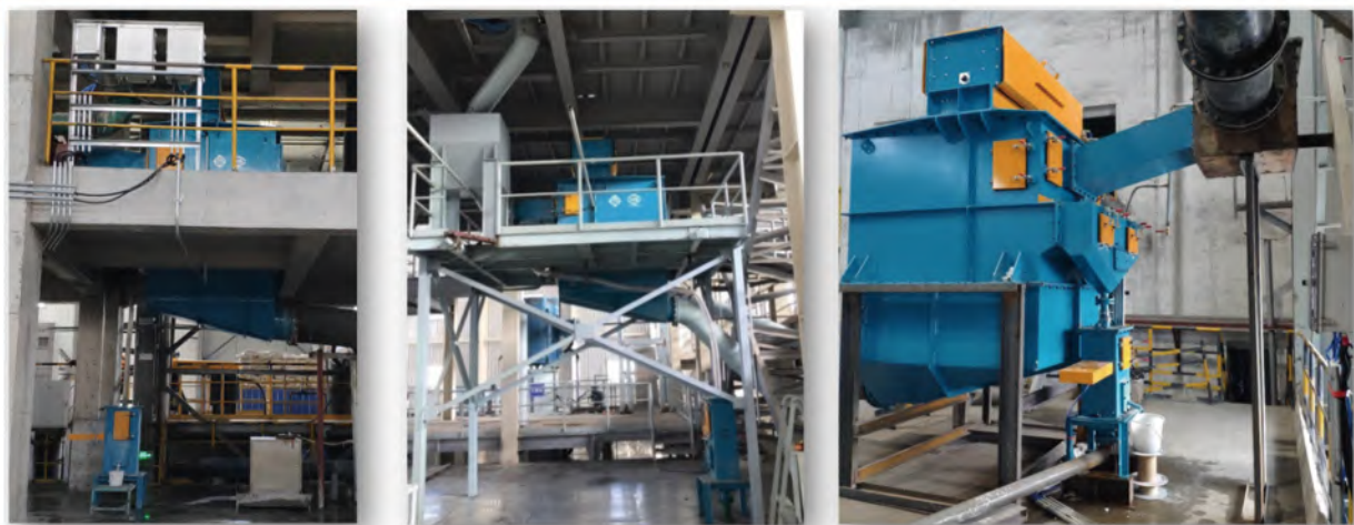
Example of BASS Series Sampler Installation in Domestic Plants
