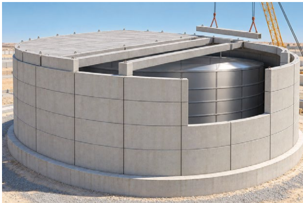
Fuel Tanks & Pumping Stations
