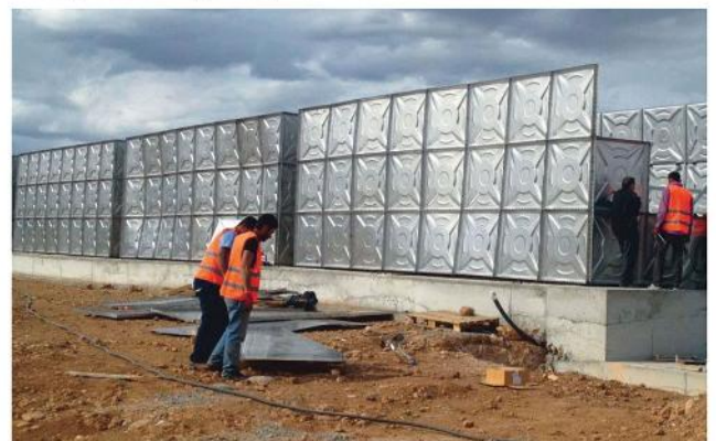
S.Urfa / Harran Refugee Camp - AISI Steel Water Tank 2400 M 3
