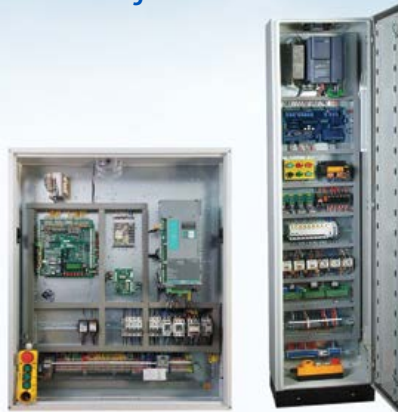
Lift VFD Panels
